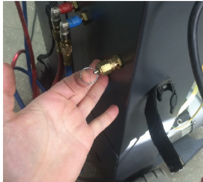
Figure 20. Discharge valve of the filling station
