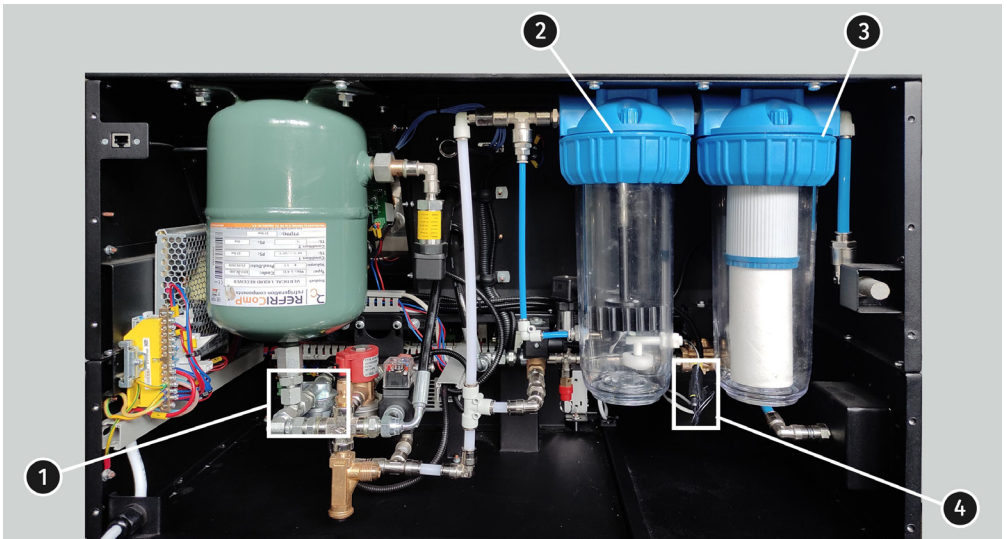
Figure 17. Location of test bench elements requiring maintenance:
